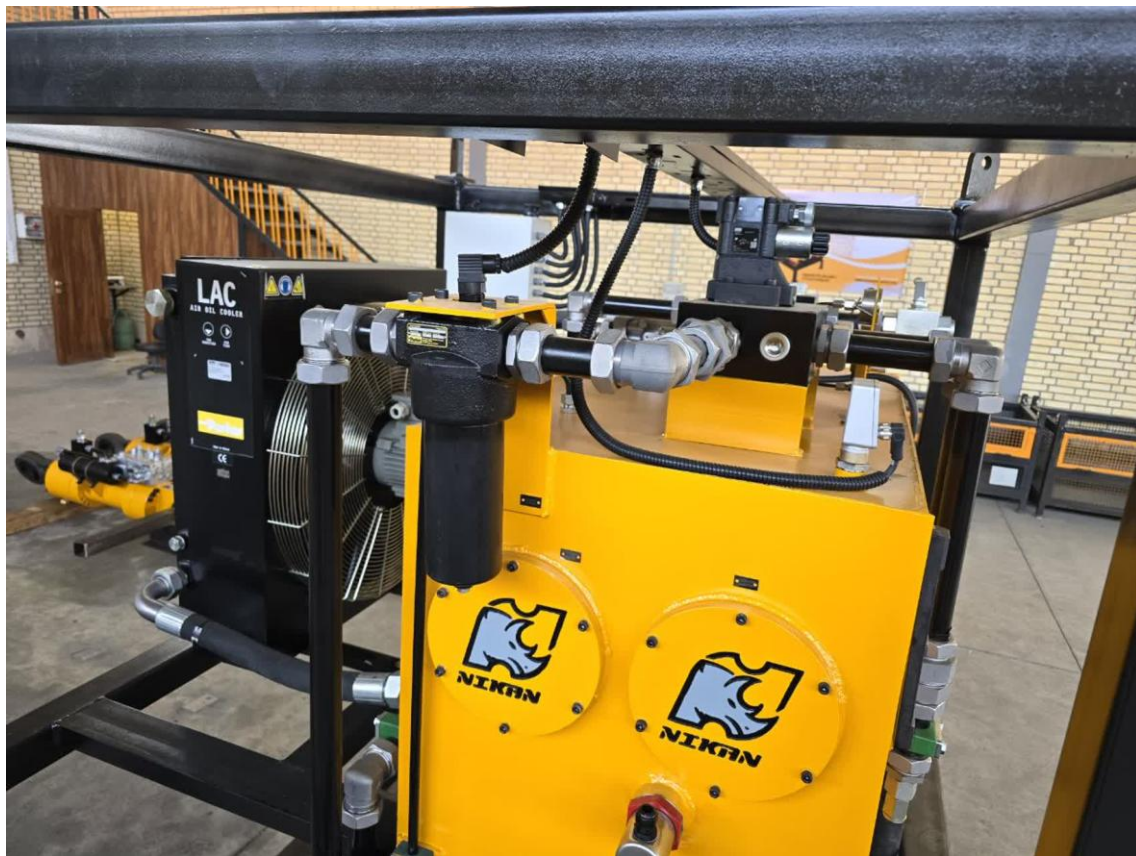
Car dumper power unit
