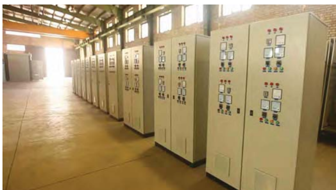
Thyristor Controlled HVAC System
