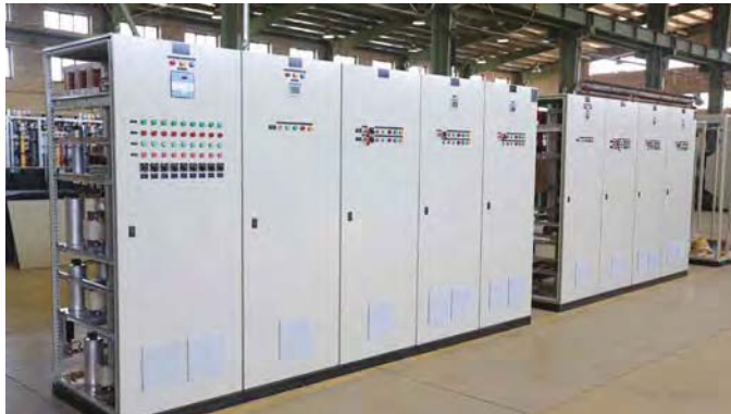
LV Capacitor Bank
