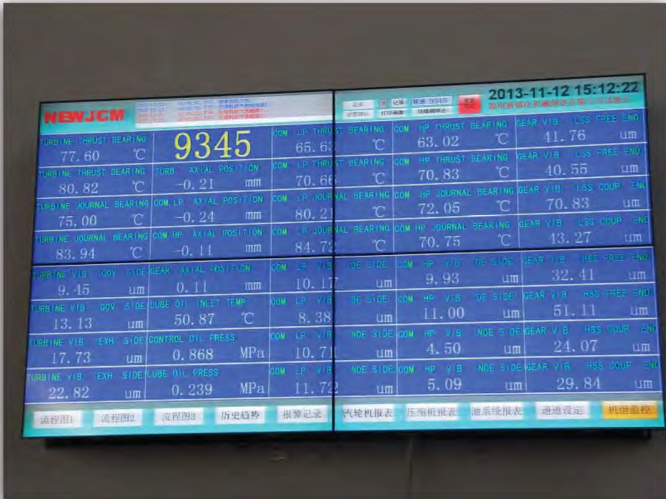
HMI Showing all important test data
