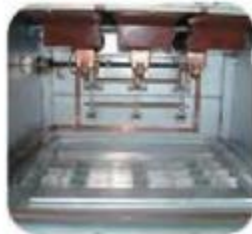
Cable compartment of RG-MEE
