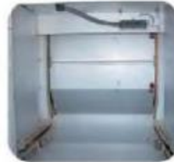
Circuit Breaker compartment of RG-MEE
