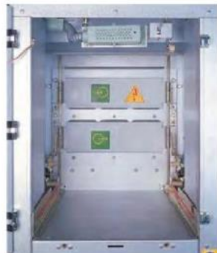
Circuit breaker compartment
