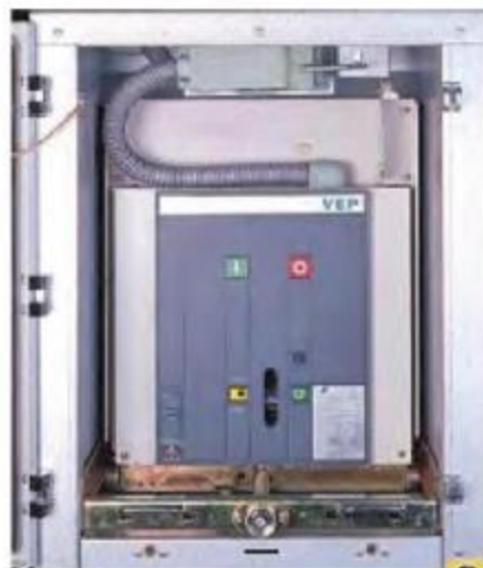
Circuit breaker in service position
