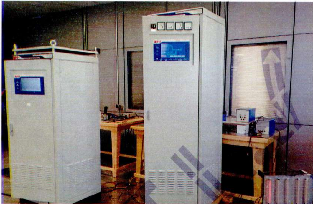
Figure 14: Conducted RF test set-up
